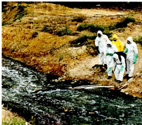
The Fire and Rescue Department hazardous materials (Hazmat) team cleaning up the chemically-polluted Sungai Kim Kim in Pasir Gudang, Johor, recently. PIC BY ADI SAFRI
